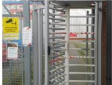
Regular cleaning of turnstile
